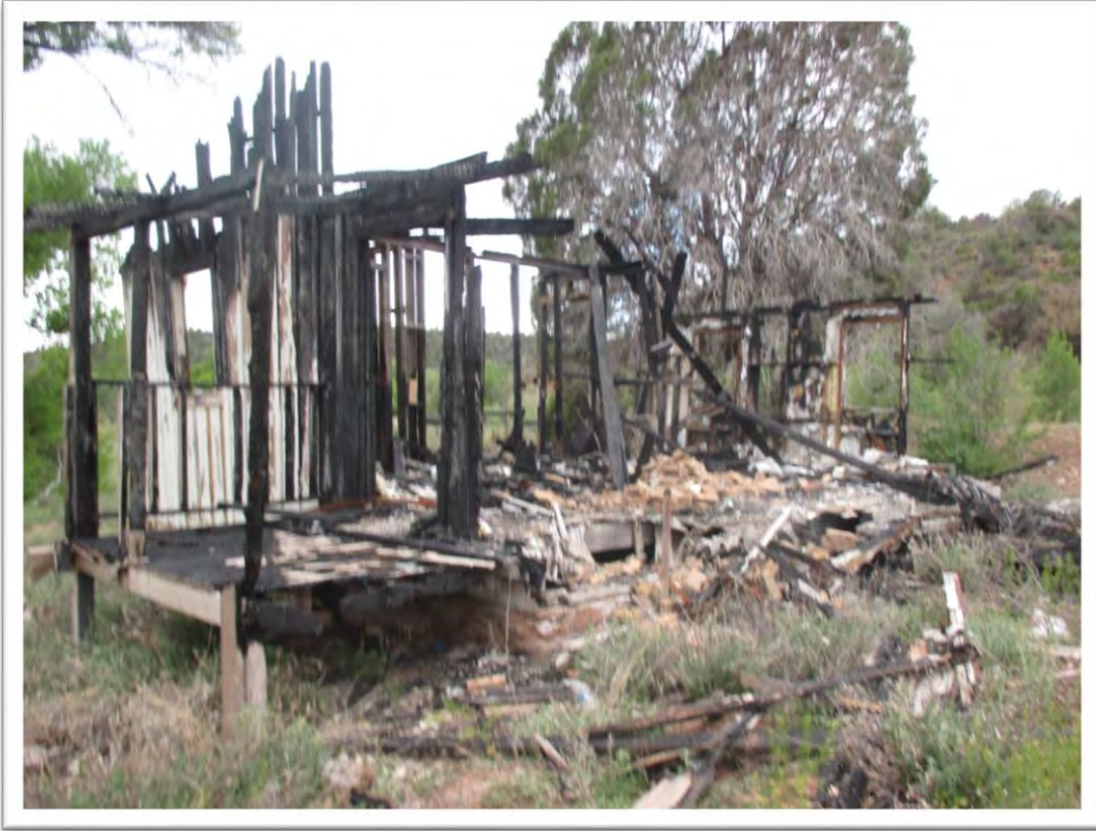
Browning site in Cibecue – burned structure, unsafe to the public.
